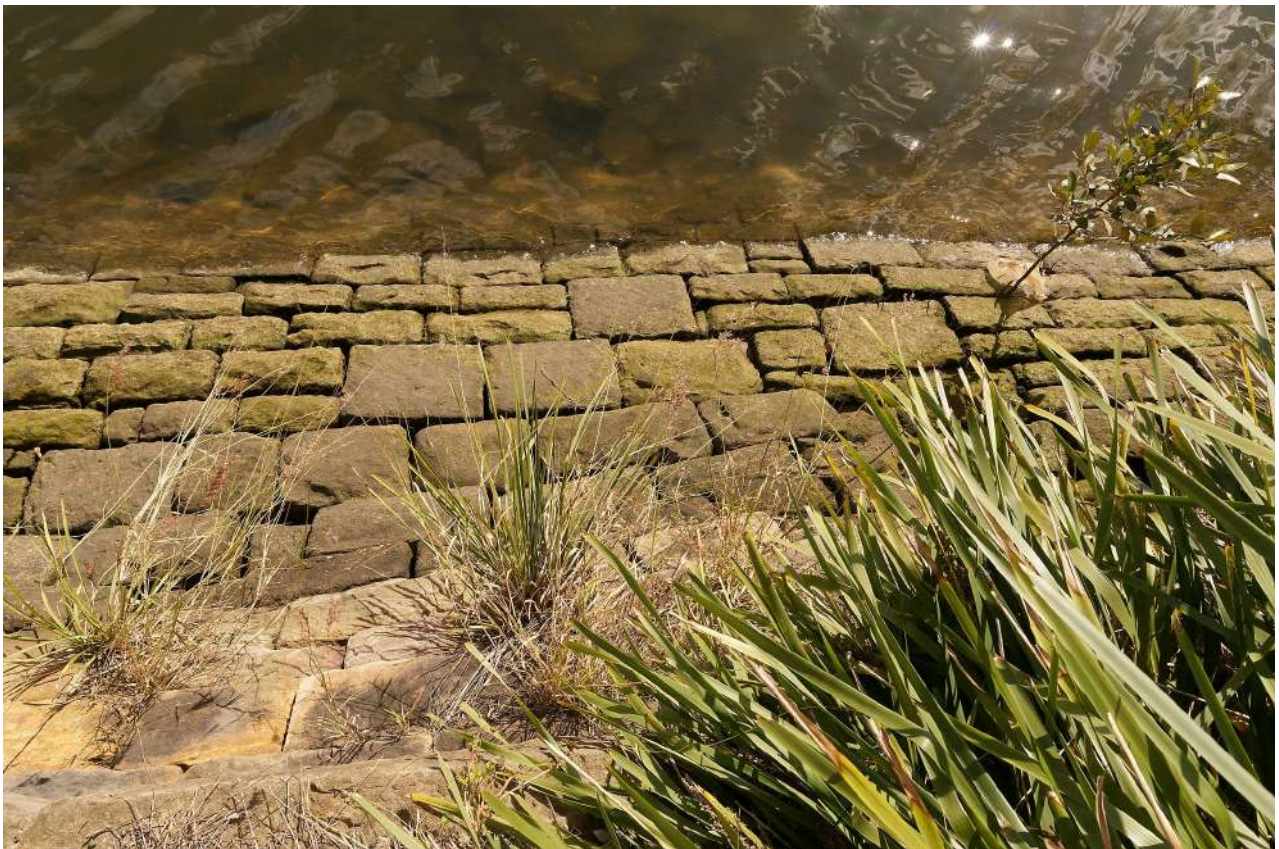
Eastern sandstone wall showing algal growth.
