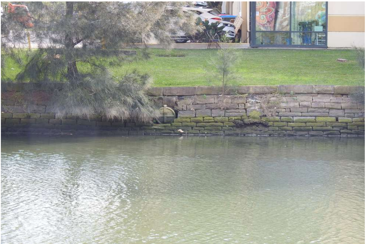
Drain in western sandstone wall with algal growth below high tide mark (closer view)
