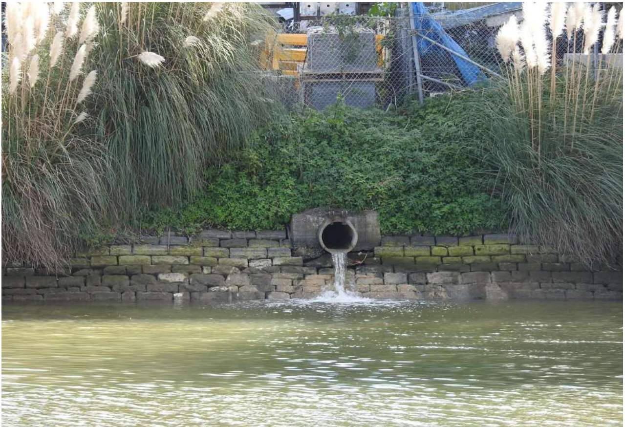
Pipe in western sandstone wall beside 32 Burrows Road, showing the absence of algae possibly from acidic drainage water.
