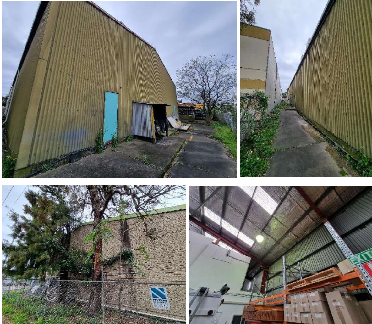
Figure I-2: Habitat investigation in large shed at 28 Burrows Rd. Insulation in shed roof.
