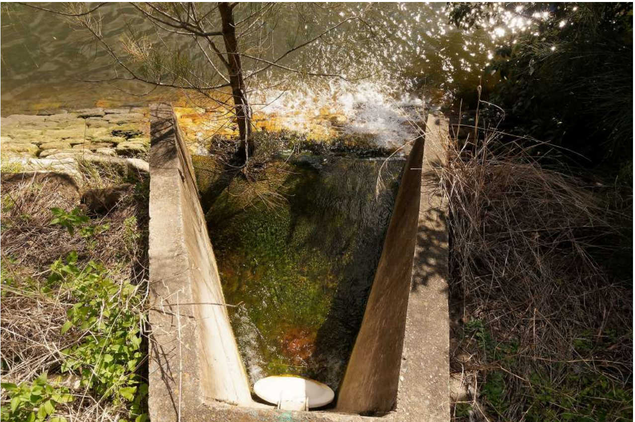
Large concrete outlet in eastern sandstone wall, rocks below outflow free of algal growth, possibly from acidic drainage water
