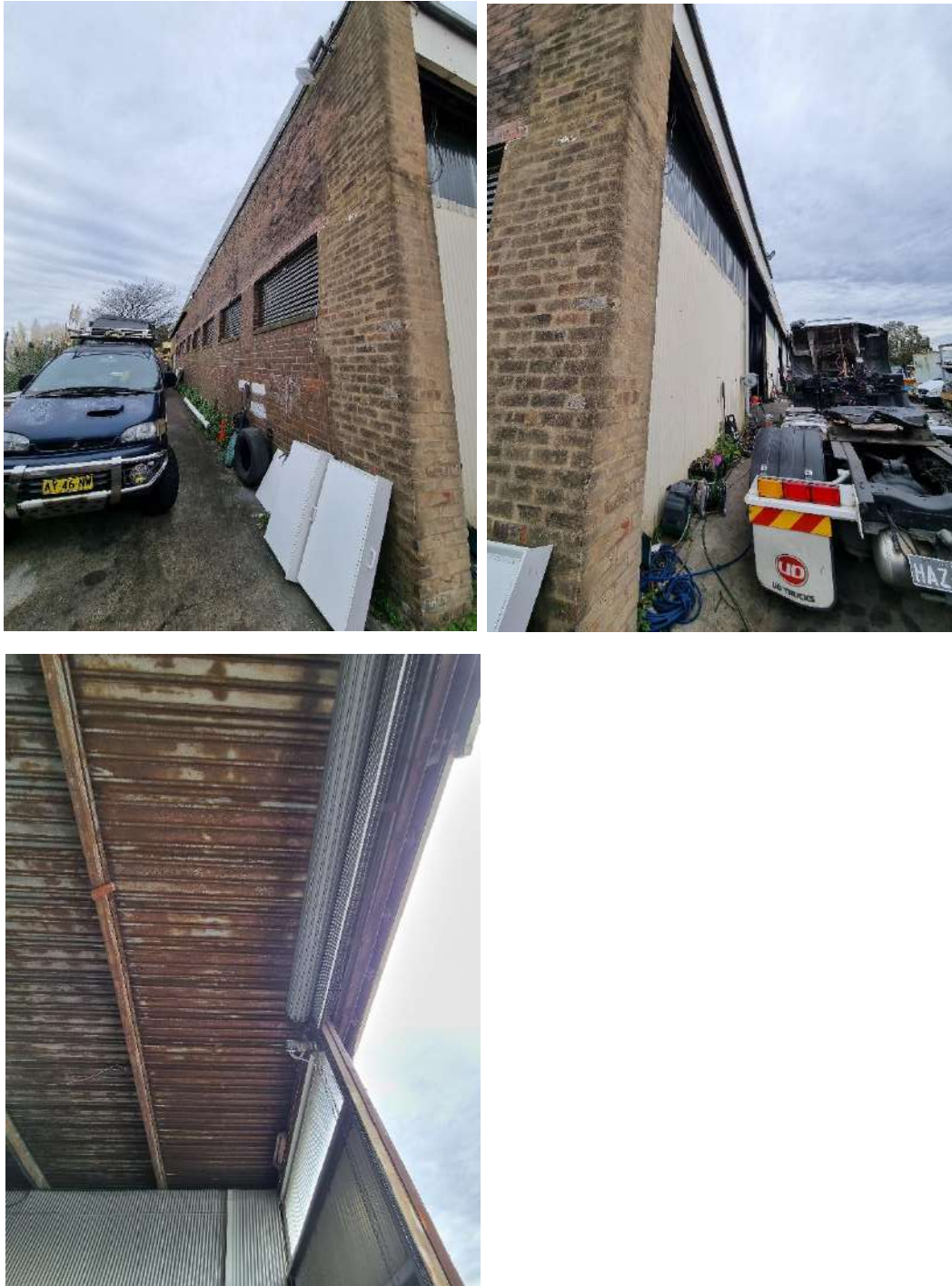
Figure I-4: Habitat investigation in large shed at 30 Burrows Rd. No insulation in shed roof.
