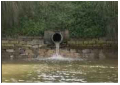
PROPOSED STORMWATER DISCHARGE TO BE CONSTRUCTED IN A MANNER TO MATCH EXISTING DISCHARGES ALONG THE ALEXANDRA CHANNEL
